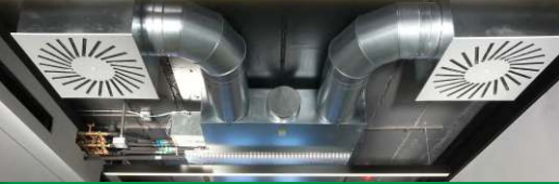
Customized HVAC Solutions
